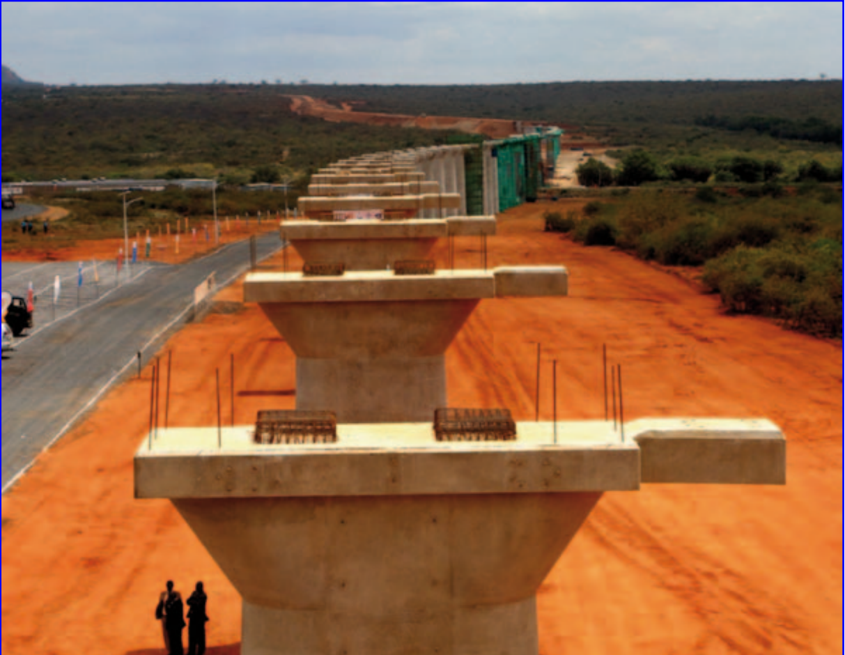
Plate 2: Piers of Tsavo River Super-large Bridge. The bridge is 1987.7m long Source: China Daily Africa, 28th May 2017 http://www.chinadaily.com.cn/kindle/2017-05/28/content_29534632.htm
